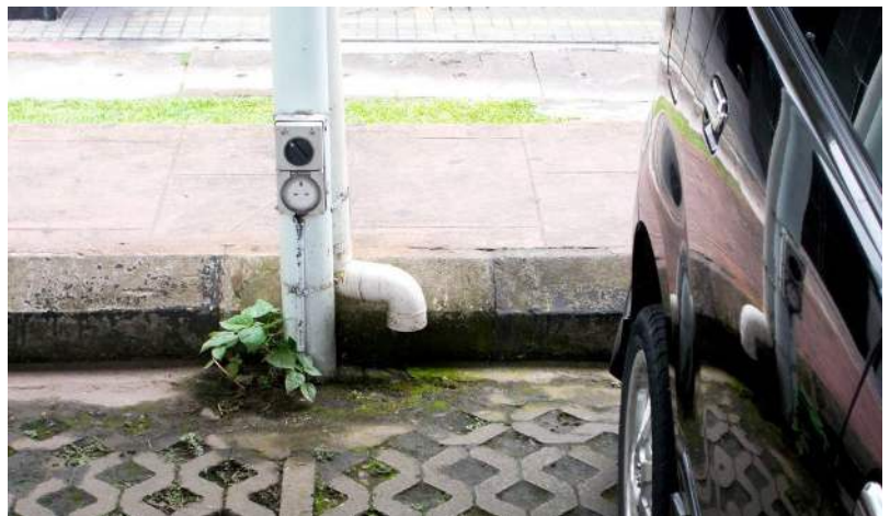
Figure 39 : Weatherproof "G-plug" at a covered parking place in Kuching, Sarawak.
