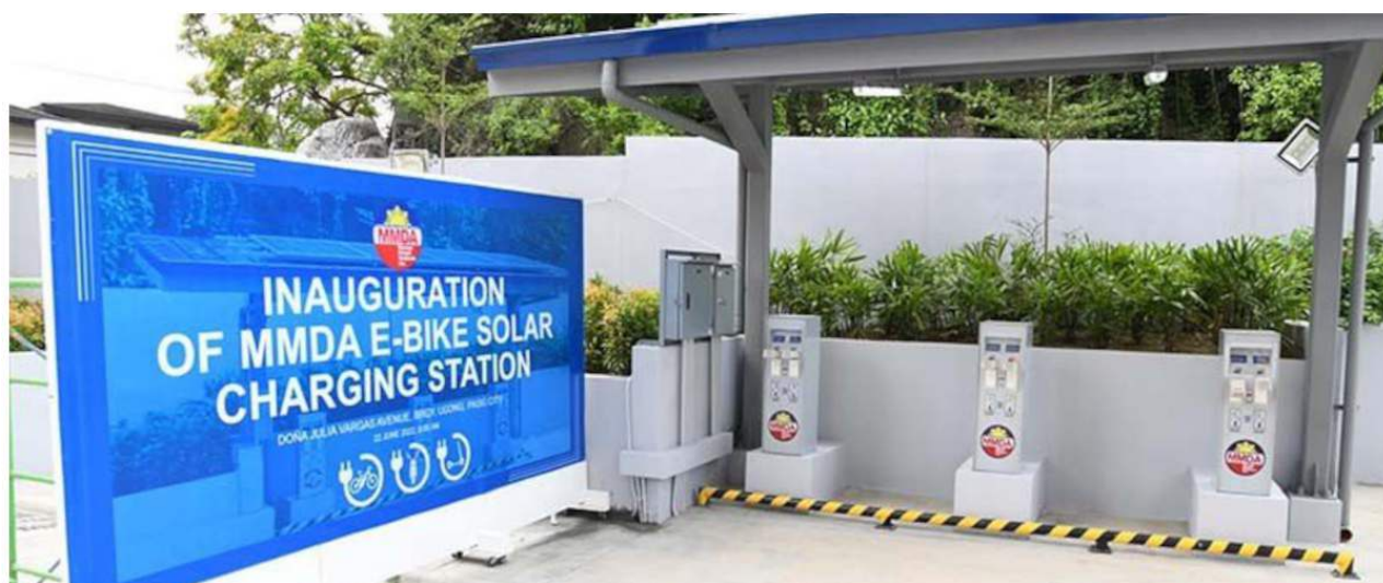
Figure 23 : Metro Manila Solar E-Bike charging station. Source MMDA
